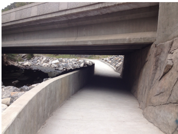
A grade-separated undercrossing using the existing slope and riverbed to pass under a roadway
