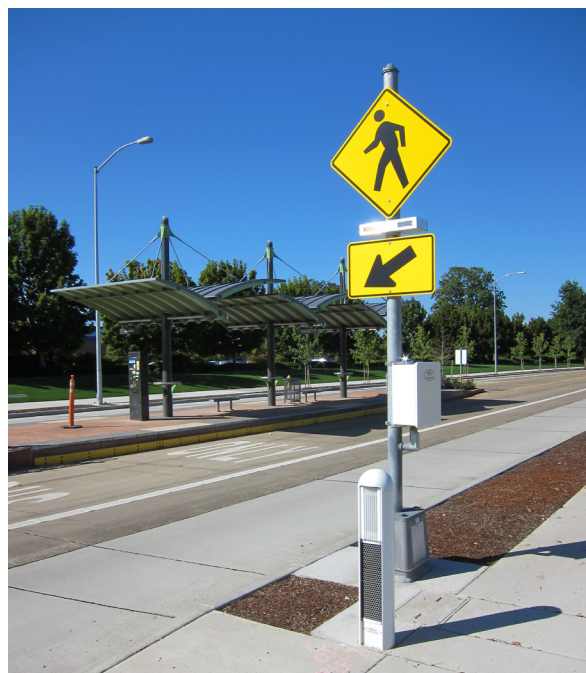
RRFB with passive detection (white bollard in foreground)
