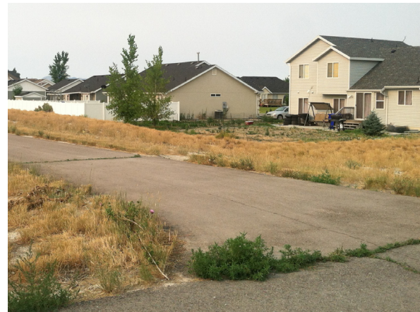
Cracks in asphalt shared-use paths can allow weeds and grasses to grow up, worsening the crack and blocking use of the path
